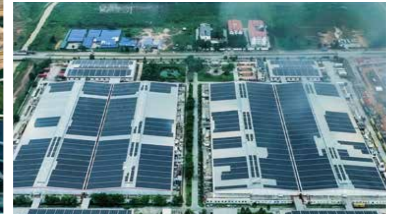
15MW ☰ D&Y Textile distributed rooftop solar generation plant 📍 Malaysia
