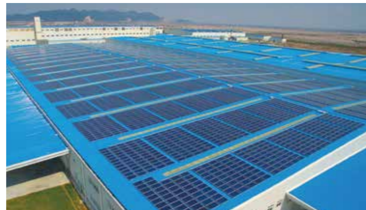
10.3MW ☰ Geely Automobile PV Rooftop Project in Linhai 📍 Linhai, Zhejiang Province, China
